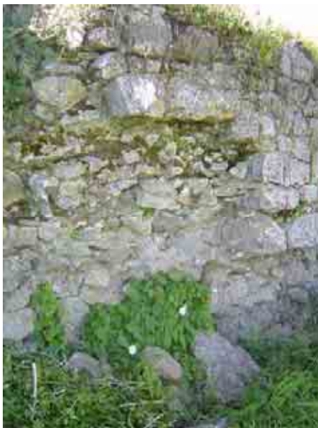
Plate 6: Loss of facing stones
