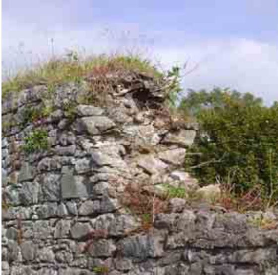
Plate 8: Unprotected wall top
