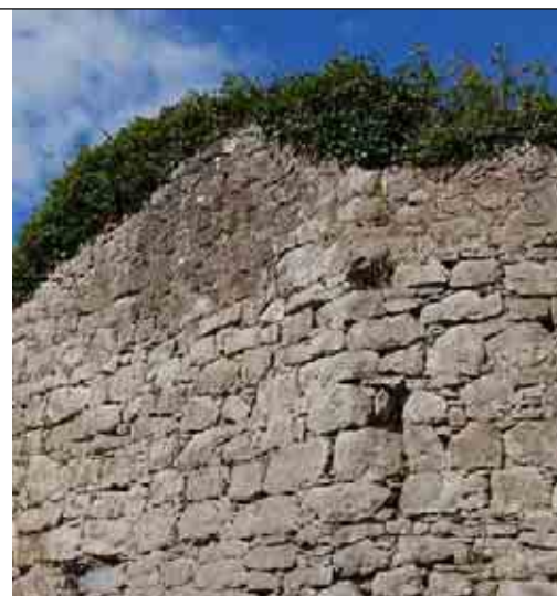
Angled facing stones at corner, with two faces, above smaller stones marking top of construction stage, looking east
