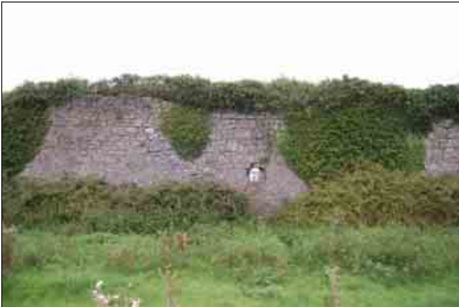
Hole in exterior of wall, looking east
