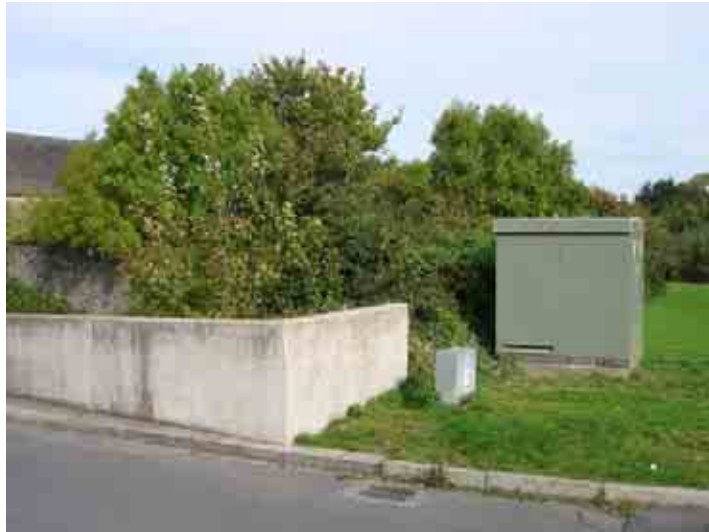
Plate 34: Inappropriate location of services
