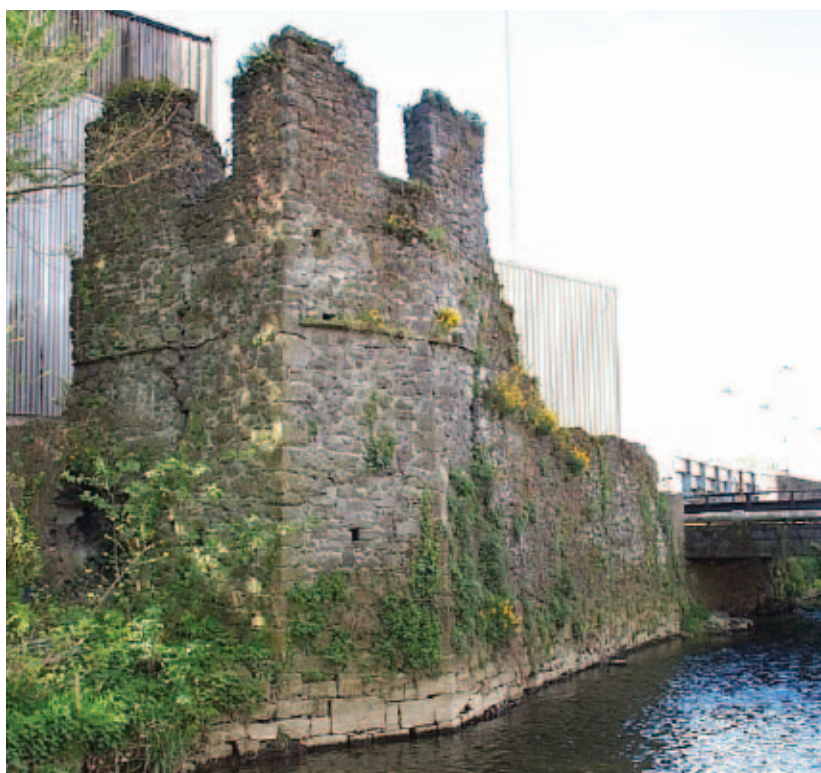
Plate 2: North-eastern polygonal tower (Evans Turret) and adjacent section of revetment wall from the north (May 2001)
