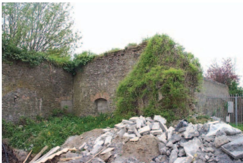
Plate 10: A length of wall, part standing and part lost, behind the Ormonde Hotel (Nos 29-32 Patrick Street)
